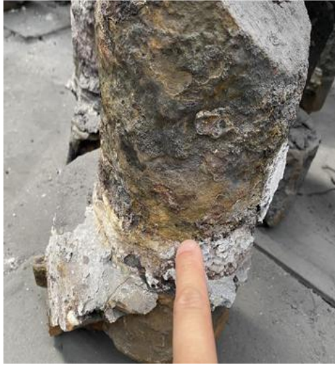
Area of Severe Oxidation on the Steel Stub
